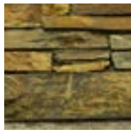
Rusty slate cement back
